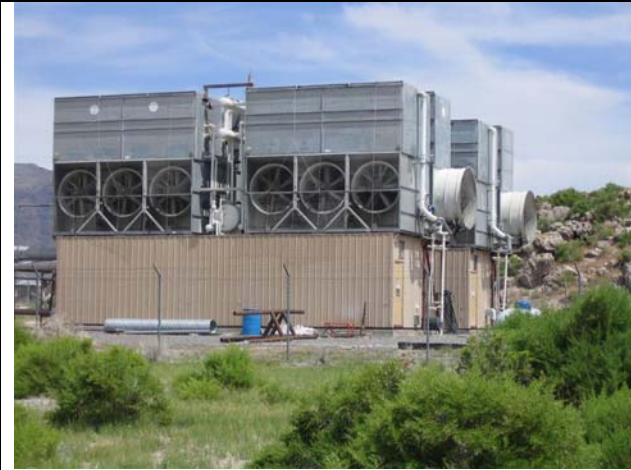
Wineagle Power Plant – only one generator is online
