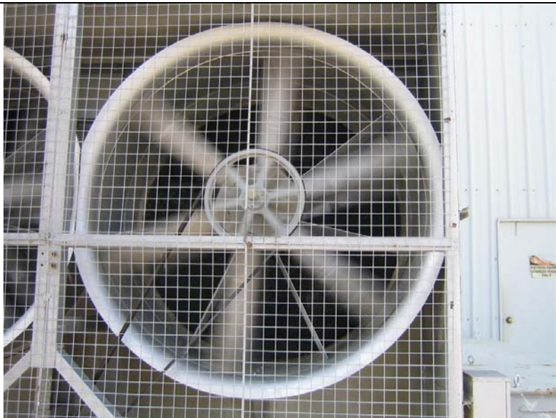
Amedee Cooling Fan in operation
