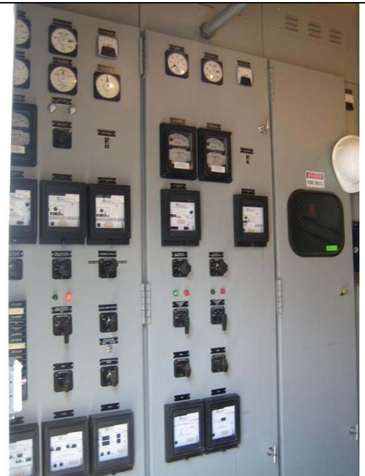
Amedee Control Room
