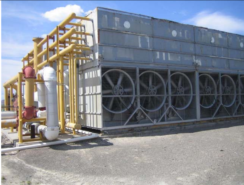
Amedee Geothermal Plant – Only one generator is online
