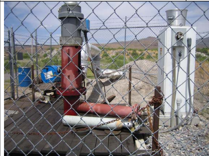
Wineagle Pump System driven by a 75 HP motor
