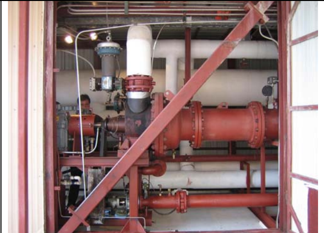
Wineagle turbine setup
